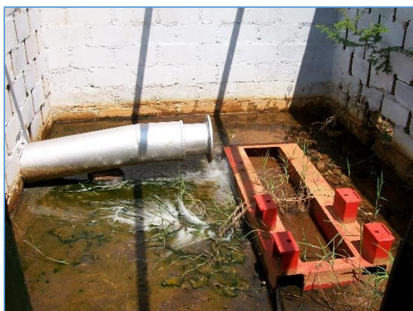
Plate 7.1: Grootfontein Irrigation Scheme in Limpopo Province: Pump plinth remaining after pump was stolen from the new pumphouse.
