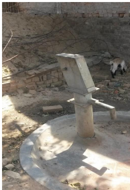
Figure 13.6 A broken water pump in Chotalakha, Jharkhand, India
