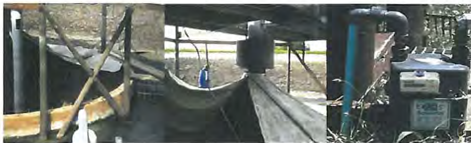
Figure 2-3: Installation of laminated reinforced PVC hood for gas capture with the nylon mesh matrices evident (left) above the fermentation pit and Flow meter (right)
