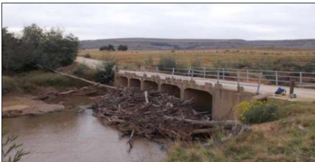
Plate 1: Bridge on the Tsitsa River near the upper Tsitsa Falls showing the accumulation of woody debris
