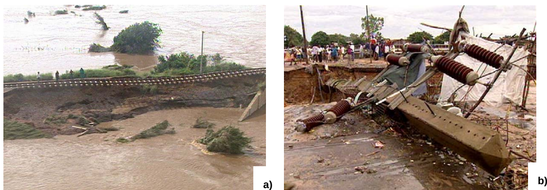
Figure 2.4: Negative impacts of the 2000 flood, Incomati and Limpopo River Basins in Southern Africa. (a) railway line destroyed in the Incomati River basin; (b) electricity supply disruption in Xai-Xai in the Limpopo River basin
