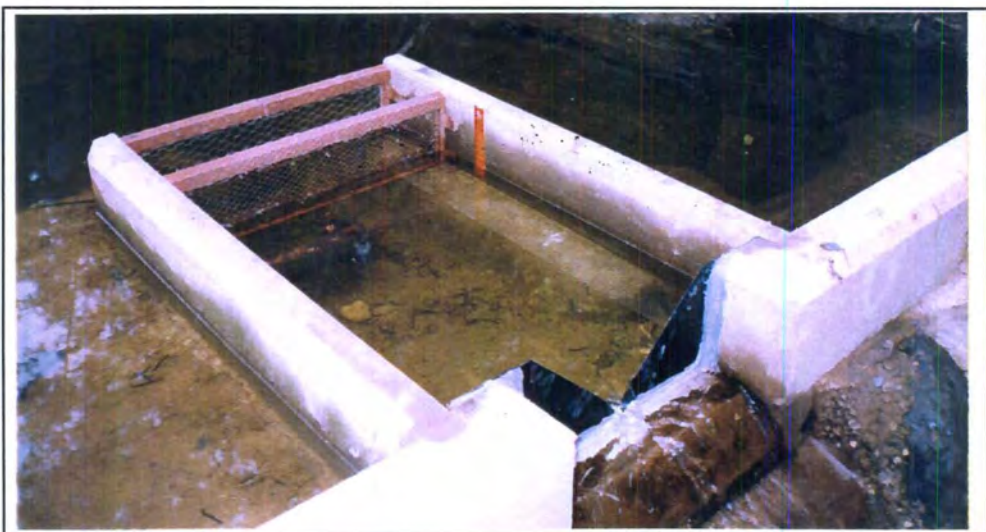
Plate 6: Weir 2 showing the design of the settling pool.
