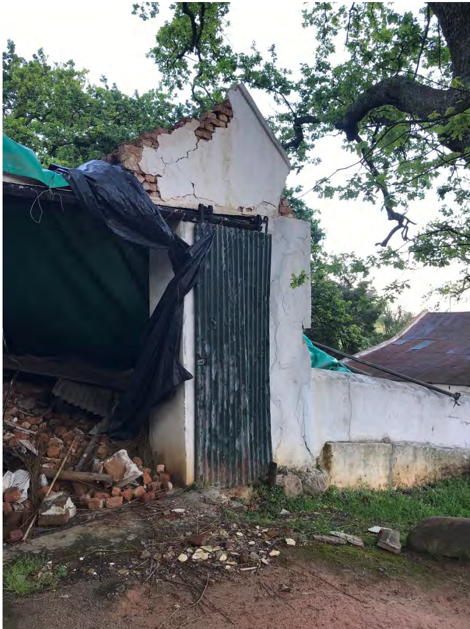
Figure 2.12: Collapsed old building on the farm. Photographed in September 2020. Photo: Daniel Retief.
