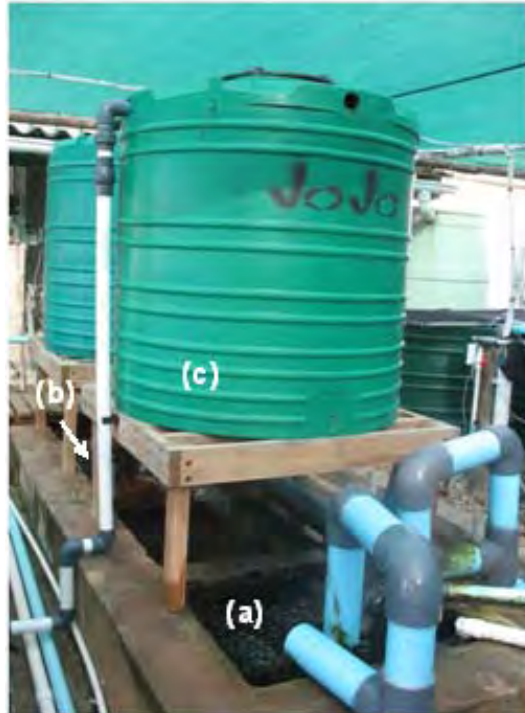
Figure 2.2. (a) The sedimentation settlement tank (1 000 L), (b) the biological filters including a submerged (1 000 L) and (c) a trickle filter (1 000 L).
