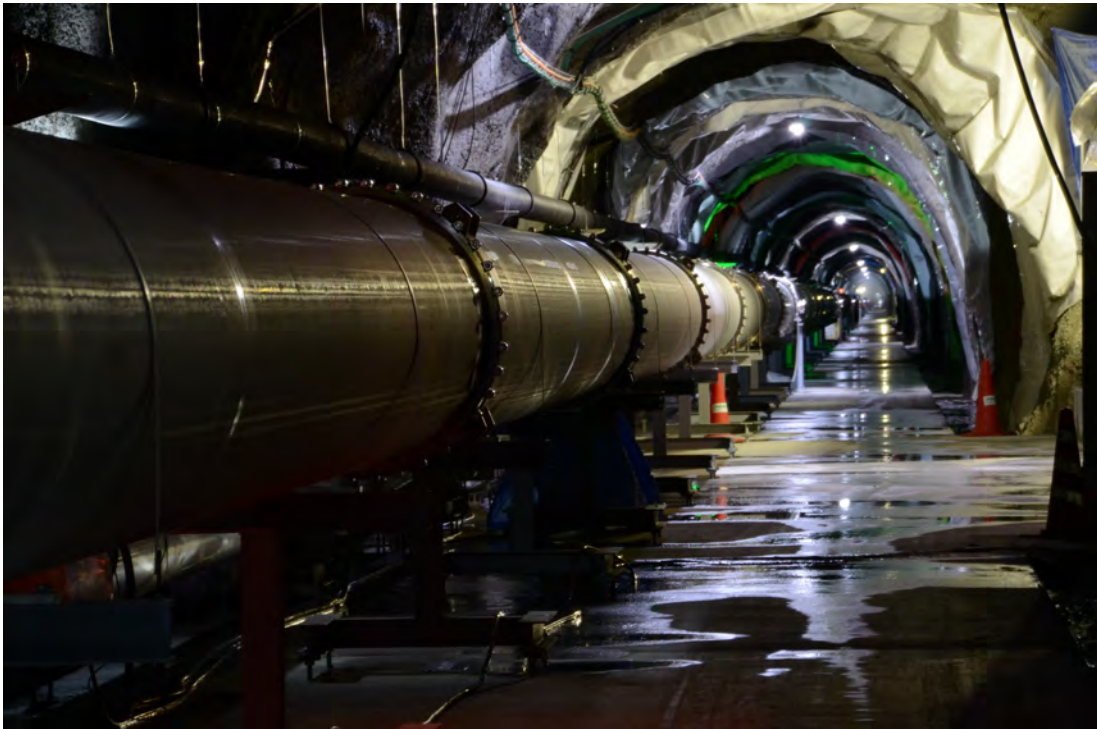
Figure 5.9: The 3 km long beam tube of KAGRA underground in the Ikenoyama mountain in Kamioka, Japan. Photo courtesy: KAGRA Observatory, ICRR, The University of Tokyo. [179]
